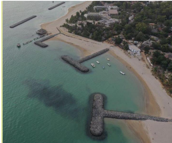
Groynes in Saly, Senegal. Photo: Senegal World Bank funded Tourism Project (PDTE)
